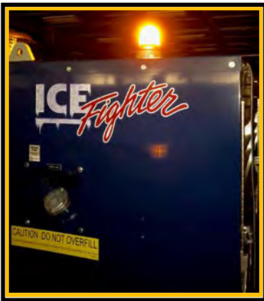
Beacon Displays Steady Amber when Keyswitch is On But Generator is not Supplying 120VAC
