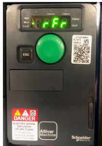
OUTPUT FREQUENCY INDICATES MOTOR FREQ. Factory Setting for VFD Display
