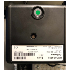
BURNER CONTROL TRIAL FOR IGNITION OR FIRING GREEN
