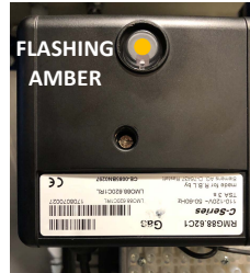
BURNER CONTROL TRIAL FOR IGNITION
