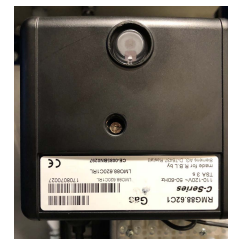
BURNER CONTROL OFF NO LIGHT
