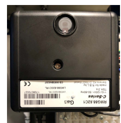
NO POWER SUPPLIED TO BURNER CONTROL WHEN LOW PRESSURE GAS SWITCH CONTACTS ARE OPEN.
