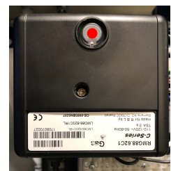
BURNER CONTROL LOCKOUT RED
