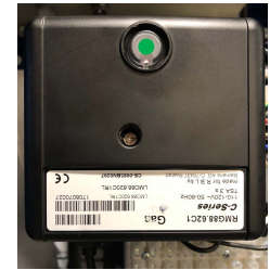
OR BURNER CONTROL FIRING GREEN
