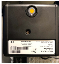
BURNER CONTROL PRE-PURGE AMBER
