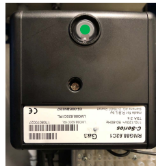
BURNER CONTROL FIRING GREEN
