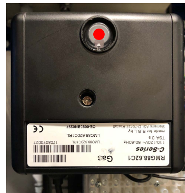
BURNER CONTROL LOCKOUT RED
