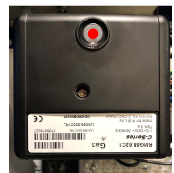
BURNER CONTROL LOCKOUT RED
