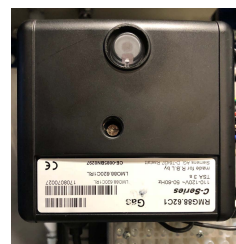
NO POWER SUPPLIED TO BURNER CONTROL WHEN LOW PRESSURE GAS SWITCH CONTACTS ARE OPEN.
