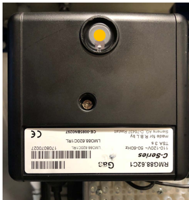
BURNER CONTROL PRE-PURGE AMBER
