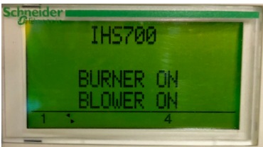
PLC DISPLAY IN CONTROL BOX
