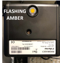
BURNER CONTROL TRIAL FOR IGNITION
