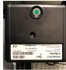
BURNER CONTROL FIRING GREEN
