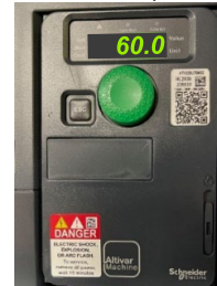
VFD - Fan is operating
