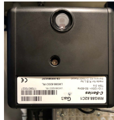
BURNER CONTROL OFF NO LIGHT
